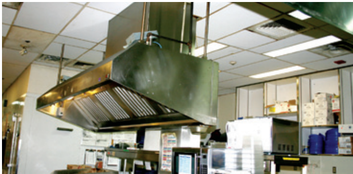
Demand control kitchen ventilation ensures fans in this hood respond to actual stove use.
