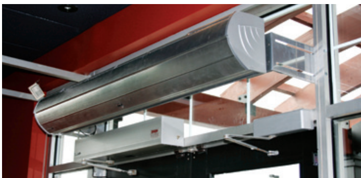
Air door at the main entrance provides comfort and heating cost savings.
